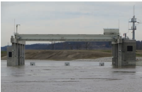
View of the overtopped powerhouse roof (tailrace side) at Cannelton on March 18.
